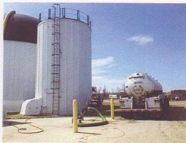
Rutland, MA Jordan's Farm Facility (Courtesy Casella Waste)
